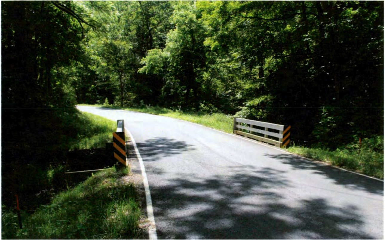
Bridge No. 121 on SR 1103 (Silvermine Road) over Silvermine Creek, view to southeast
